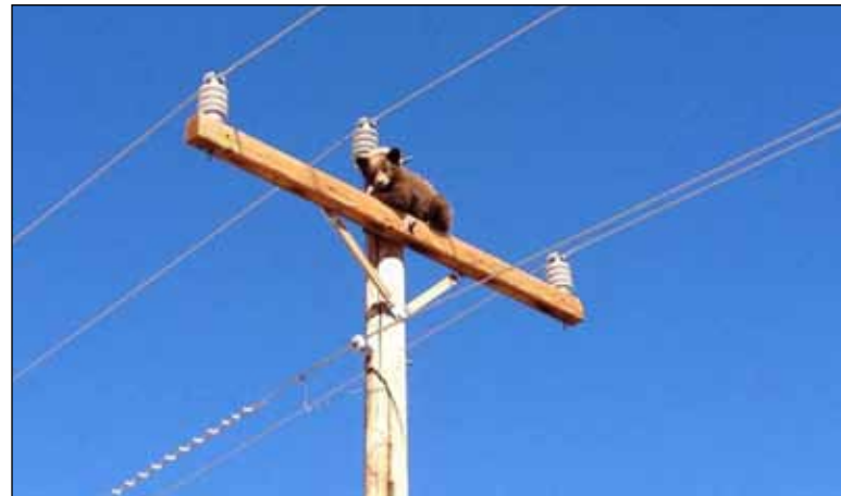
ABOVE: A Benson co-op crew discovered a bear cub on a distribution pole crossarm in the fall of 2012. They notified Sarah Sager (at that time SSVEC's environmental services specialist) who contacted Arizona Game and Fish. The cub was too young to be tranquilized, so linemen used a bucket truck and a pole noose to safely lower the bear to the ground.
