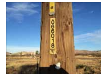
Each SSVEC power pole is labeled with a location number. It is six digits arranged vertically on a yellow strip. Provide this number when you report a problem.
