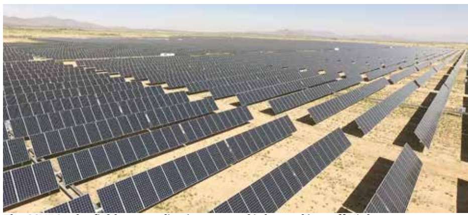
The SSVEC solar field went online in 2016 and is located just off Highway 191 near Cochise. The field generates about 20 megawatts of electricity and contributes to the Cooperative energy mix.
