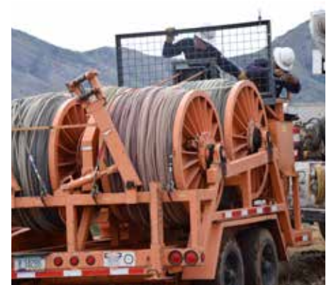
From left, Grant McCune and Jose Salinas operating the four-drum rope puller.
